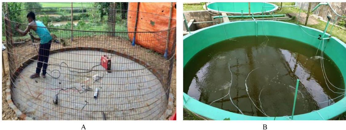
Fig. 3. BFT tank construction process using wire mesh (A) and concrete material (B). Picture courtesy of Mr. Debtanu Barman (CEO Aqua-Doctor Solutions Co. Ltd, India).
